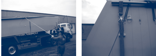
Figure 7.3.2.c. – Closing the roof sheet, Dawnbarn type, with pull back cord and tightening the sheet
